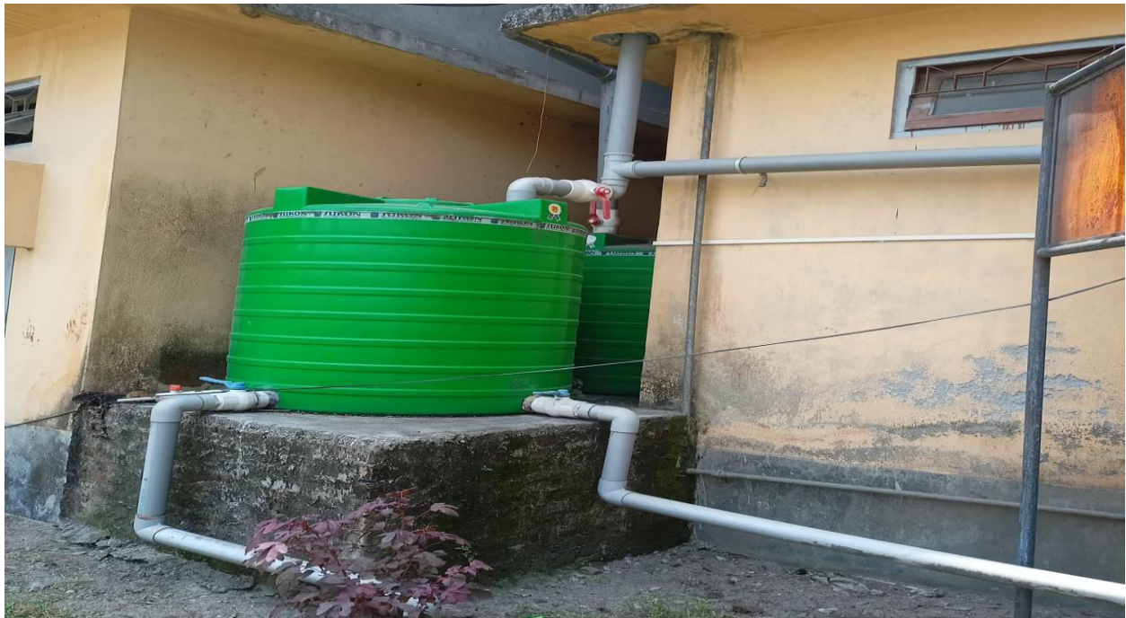
Rain Water Harvesting Unit 1
