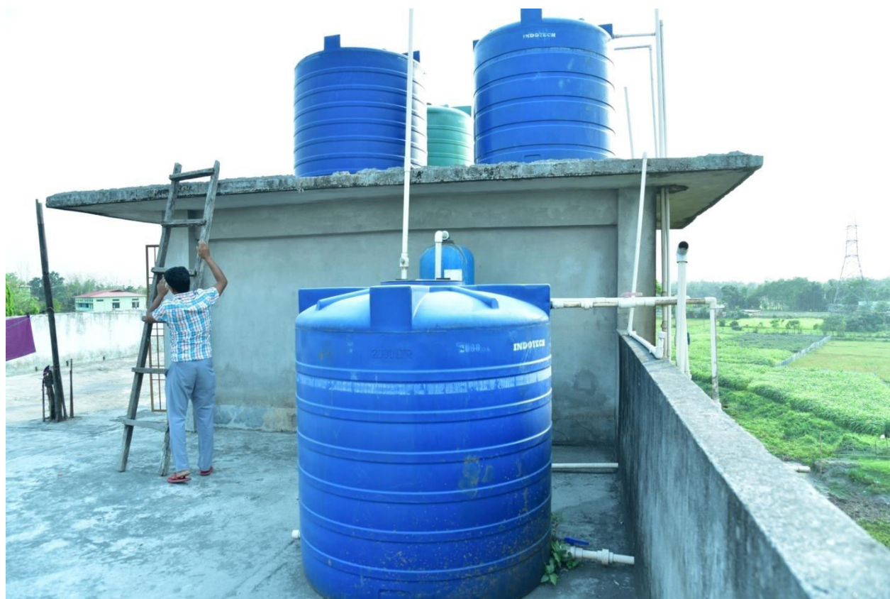
Rain Water Harvesting Unit 3
