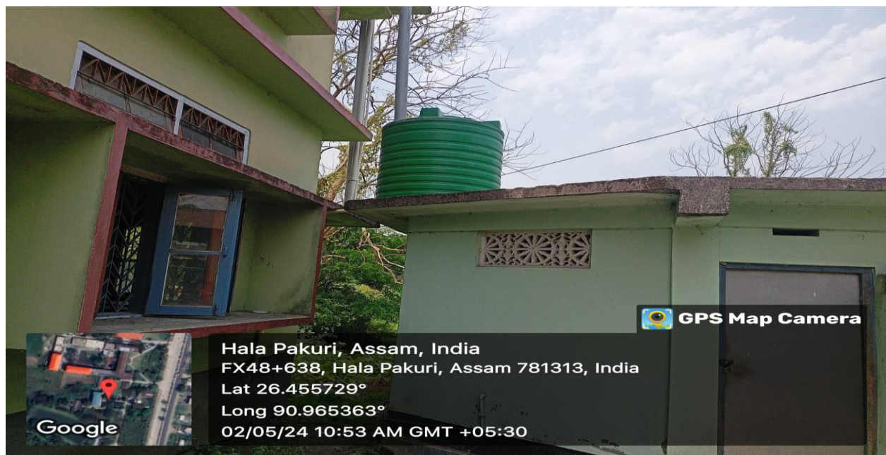
Rain Water Harvesting Unit 2
